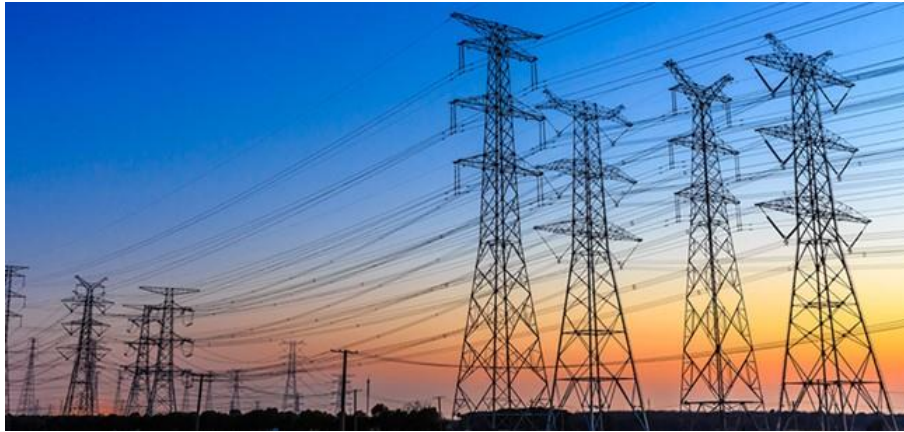
Figure 10: Typical View of an OHTL
