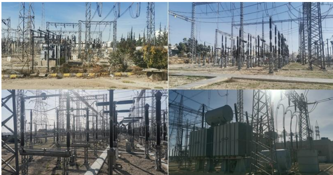
Figure 8: Typical View of a Substation
